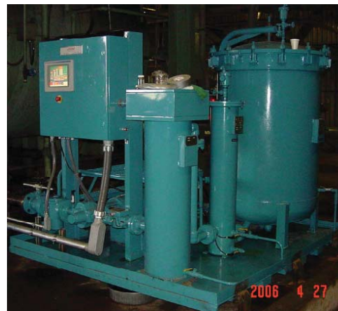
Model KL30 at Power Plant in Oklahoma
